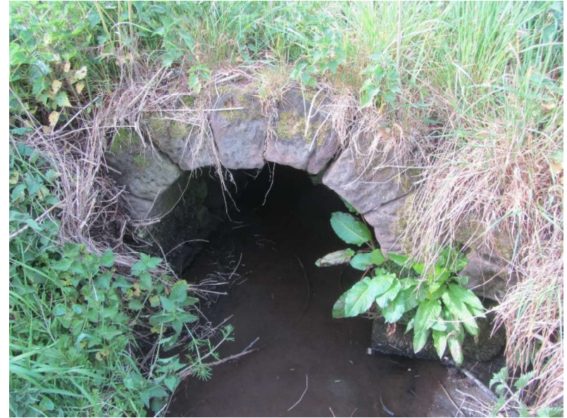
Plate XII: The fourth bridge to the south of Hooton Road in Childer Thornton. Its design is identical to the previous bridge. The arch is three feet across, which gives some indication of the narrow width of the brook it crosses.
