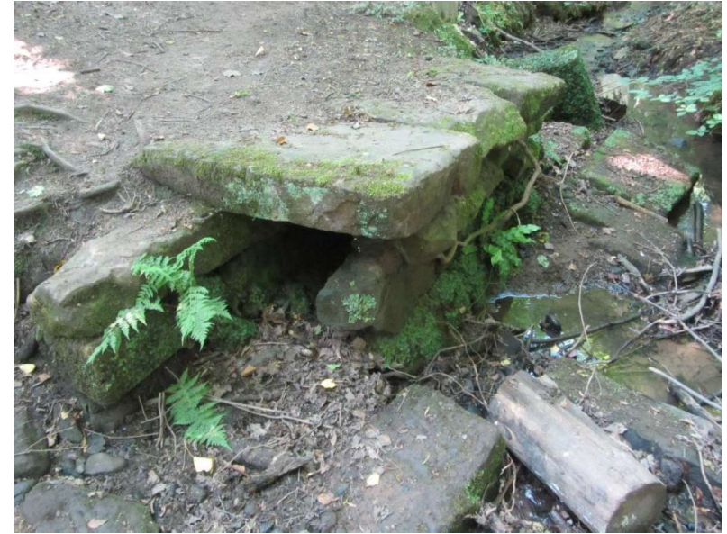
Plate VIII: The remaining section of the Bromborough bridge, as seen when looking downstream. The two sandstone piers which support the slabs are now visible. The pier in the foreground extends well past the extant slabs, showing the bridge to have once been wider. In the background some slabs which probably once formed the top of the bridge, may be seen lying out of context in the watercourse.
