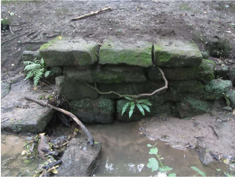
Plate VII: Bromborough clapper bridge as viewed from the bank of the stream it once crossed. The three large sandstone slabs are only wide enough to cross half of the stream. Two piers, which have now entirely disappeared, must once have supported a further row of slabs in the foreground.
