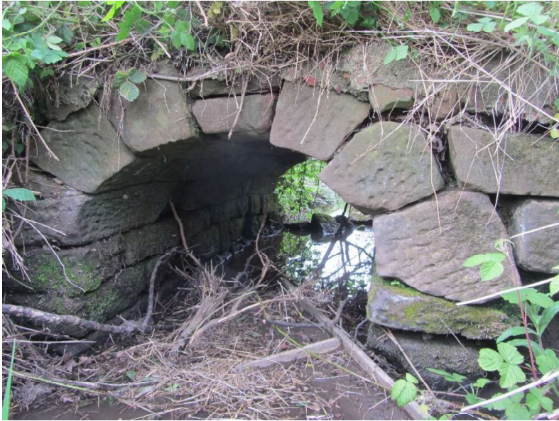
Plate XI: This is the third arched bridge to the south of Hooton Road. It is also the first intact example, for only a few courses of stone remain of both the previous bridges. The stonework inside the arch fits together beautifully and is very well-dressed.
